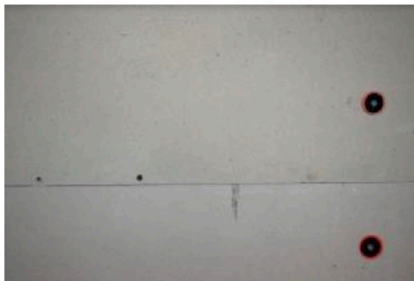
Connection between Mute 23 panels and DCIox
